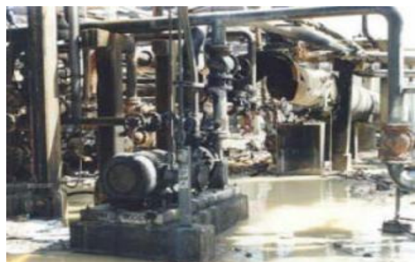
Figure 2. GP 905 Heat Exchanger of Longford Gas Plant
